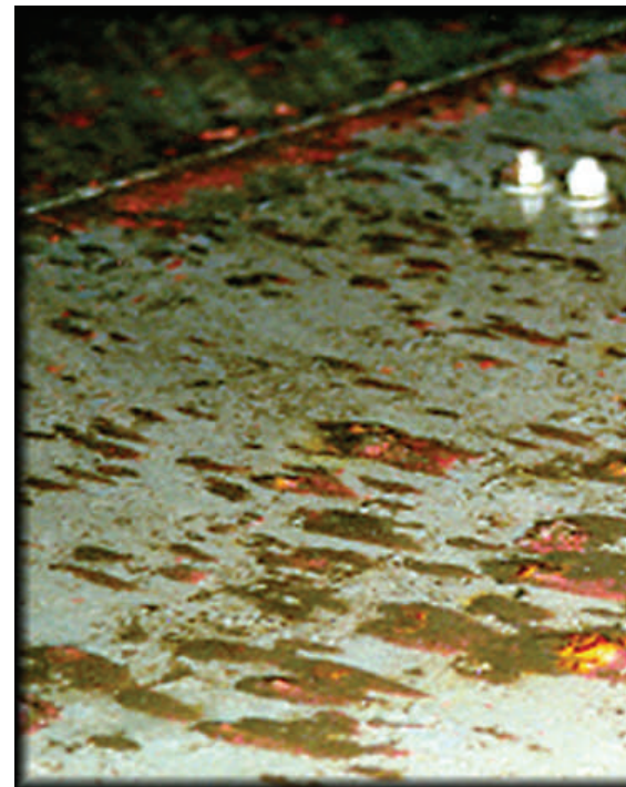
Tower basin with typical reddish to yellow growth.
