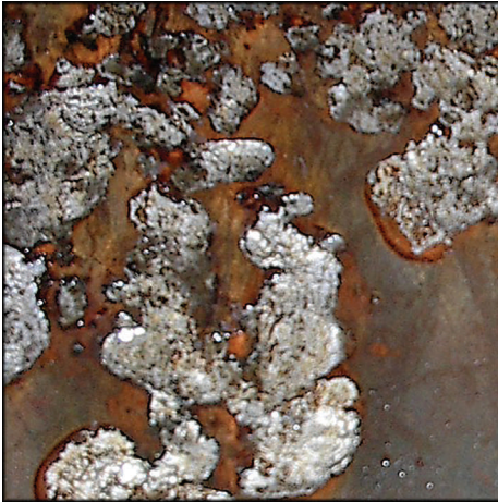
When nodules are removed, deep pits are revealed. If left unchecked, SRB-caused corrosion can penetrate a tower basin in months or even weeks
